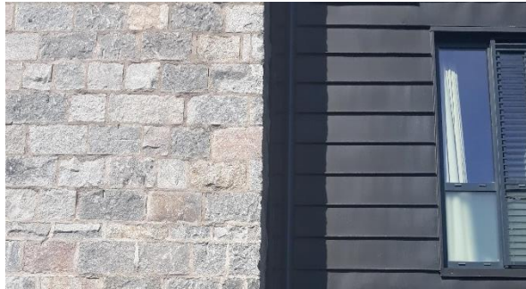
The jointing in the metal cladding at Causewayend ties in with the coursing of the adjacent granite.
